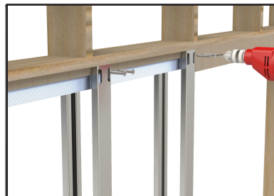
Stud frames, floor plates and door guides
